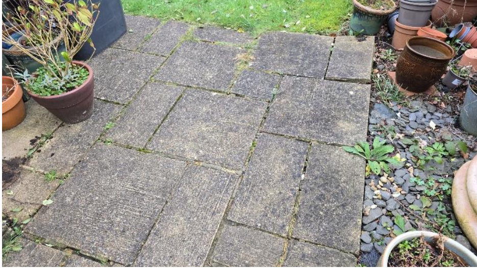
Repairs required to patio
