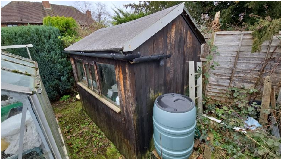
Dilapidated shed no access
