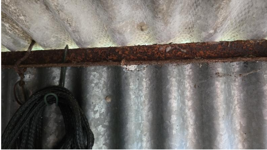
Corrosion to steel frame
