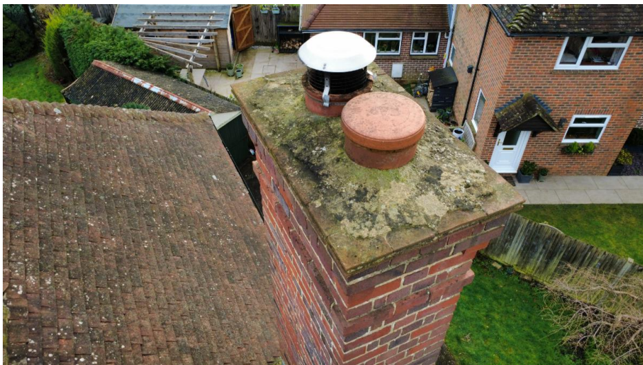
Flaunching replacement required
