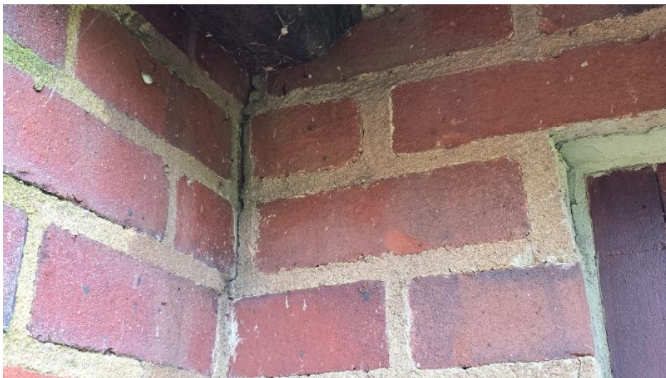
Vertical cracking where porch adjoins main house
