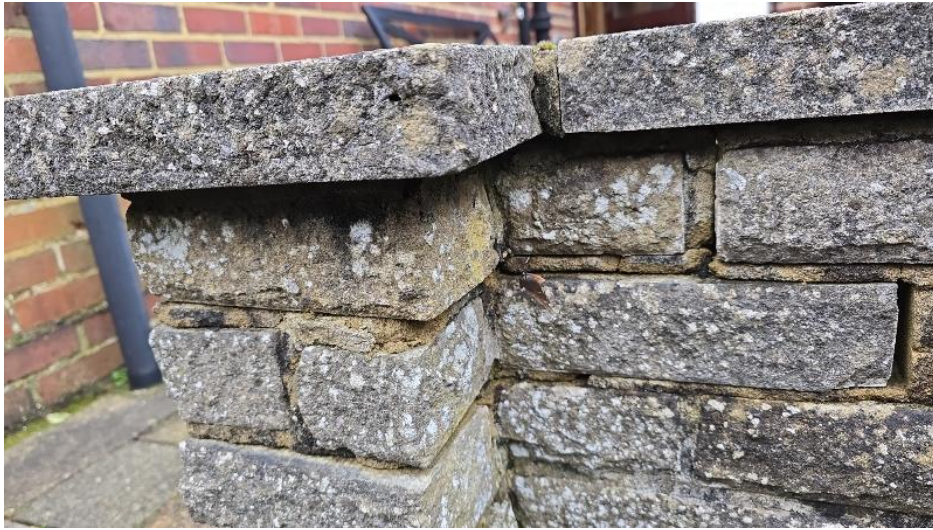
Structural movement/impact damage to low level wall off garage
