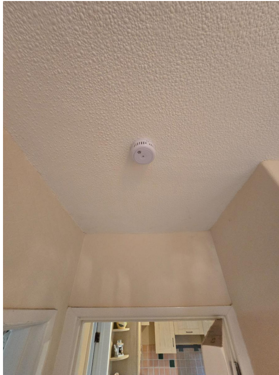
Battery powered smoke alarm ground floor hall
