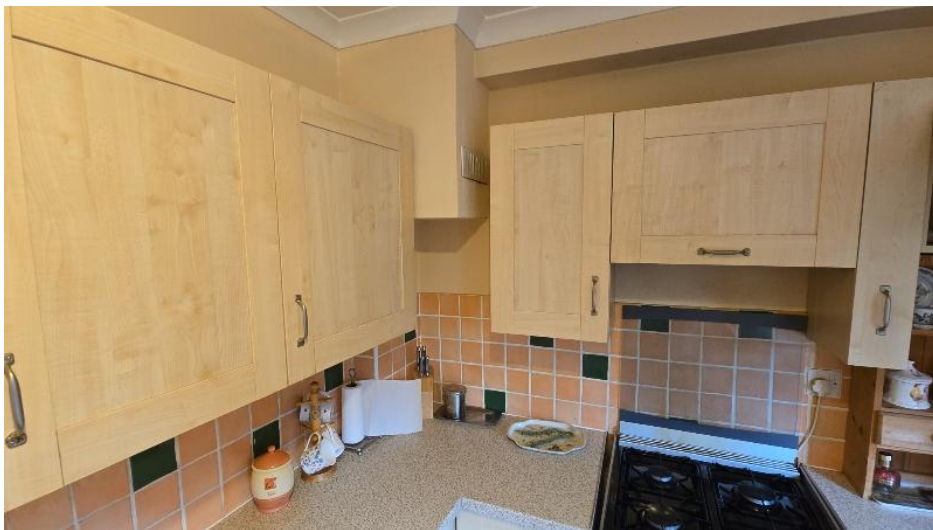
Shared party chimney part visible in kitchen no supports visible and may/may not be concealed
