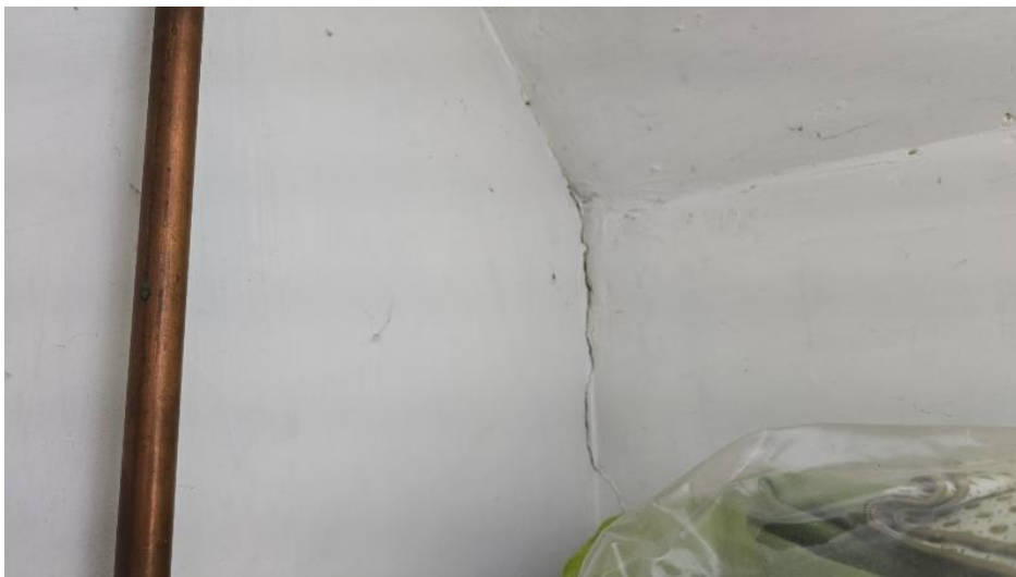
Cracking to external airing cupboard wall
