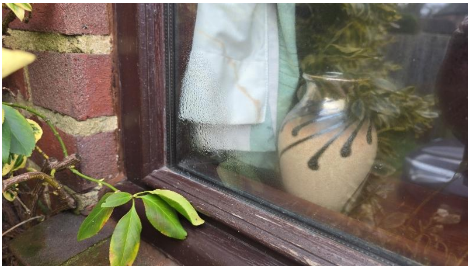
Failed double glazed seal units stairs window
