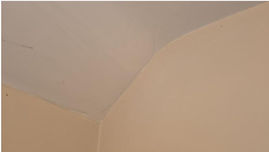
Cracking to ceiling in bathroom
