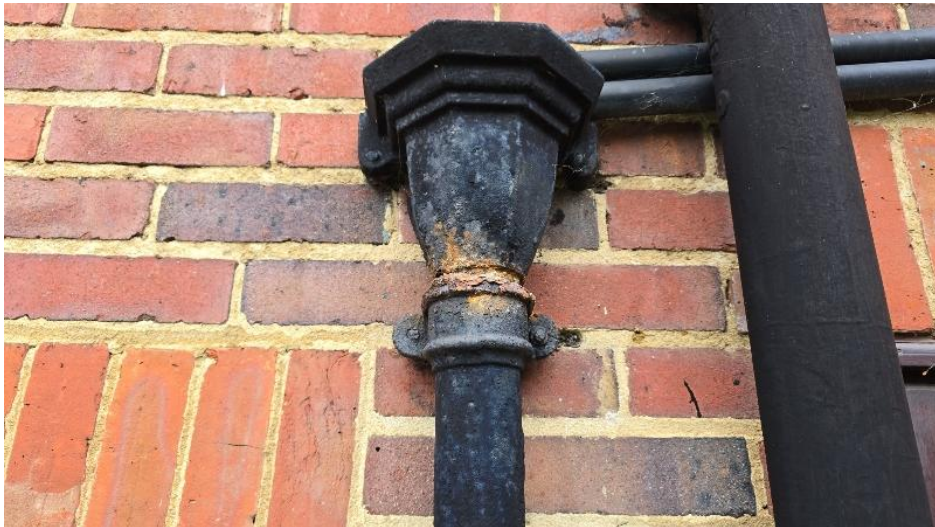
Cast iron downpipe and hopper repairs required
