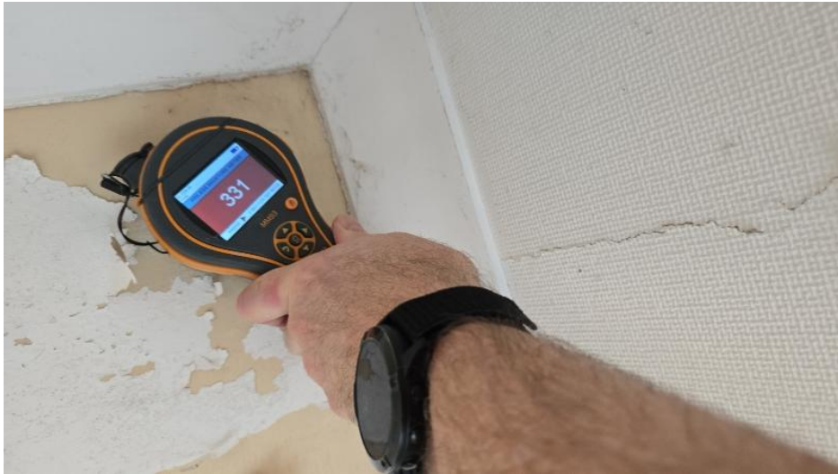
Damp to Porch ceiling
