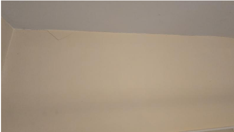
Cracking to bathroom party wall
