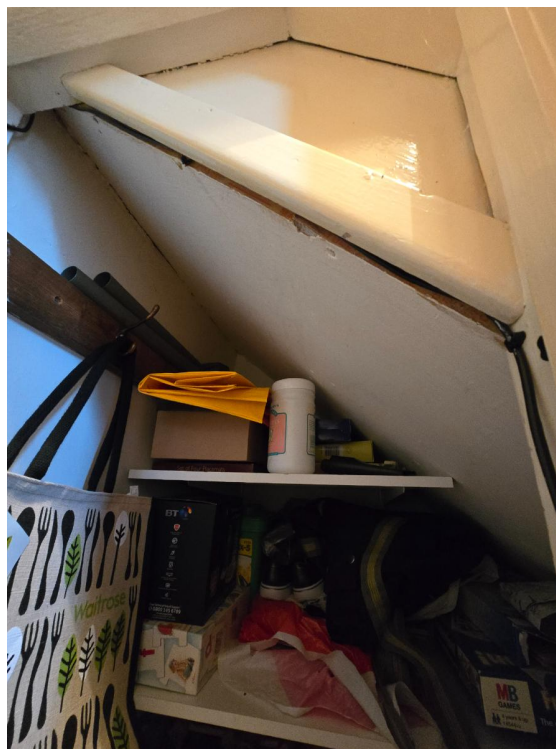
Presumed asbestos to soffit of understairs cupboard
