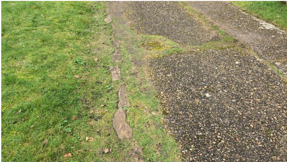
Driveway repairs required
