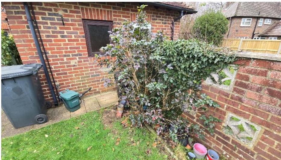
Vegetation to be removed to ascertain extent of remedial works to wall
