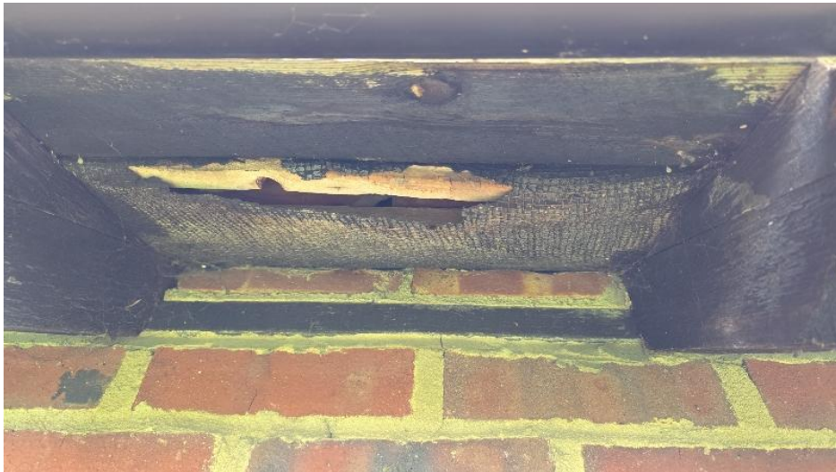
Defective timber to eaves. Will require removal of courses of tiles to rectify.
