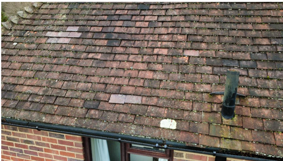
Spalled, slipped and broken tiles. Evidence of recent repairs
