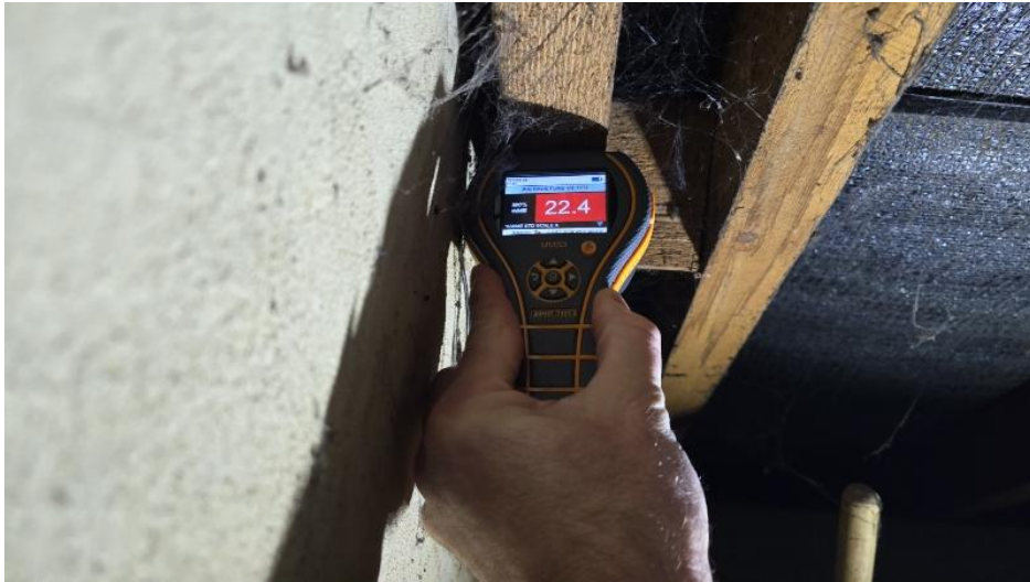
High moisture reading to shared chimney timbers
