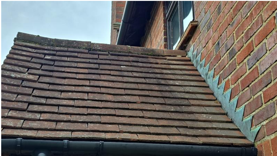
Loose ridge tiles to porch
