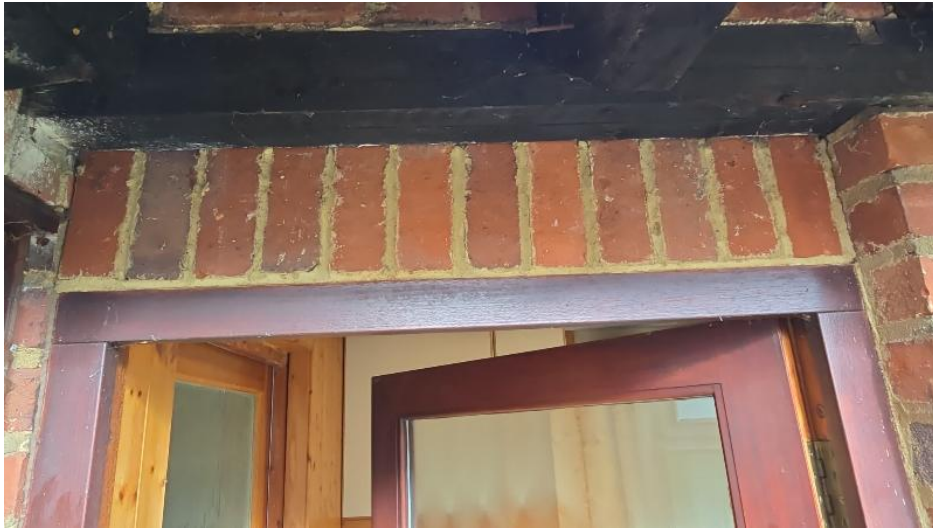
Cracking either end utility lintel
