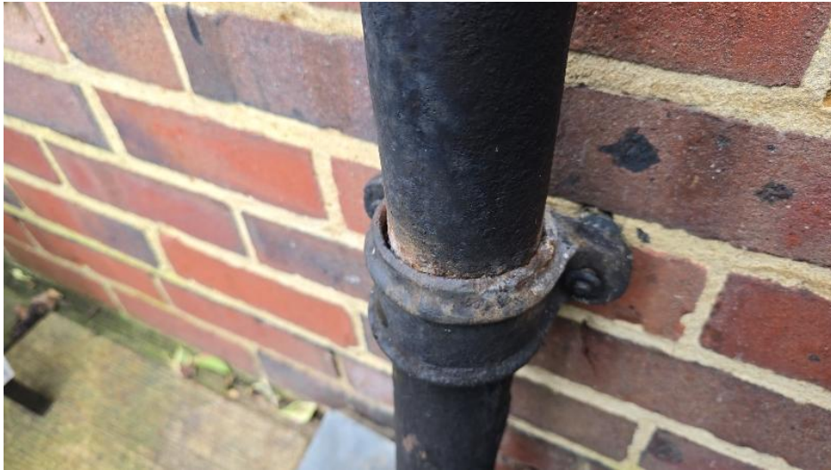
Cast iron downpipe and hopper repairs required
