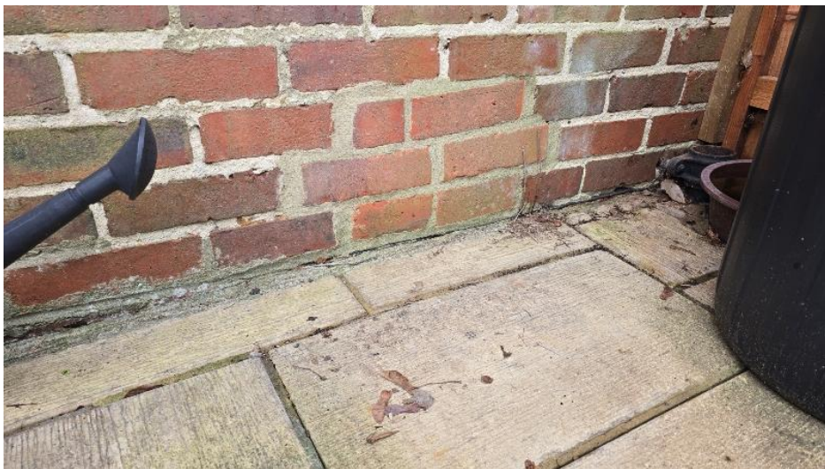
External ground level off rear needs reducing
