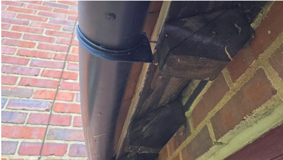
Defective timber to underside of eaves
