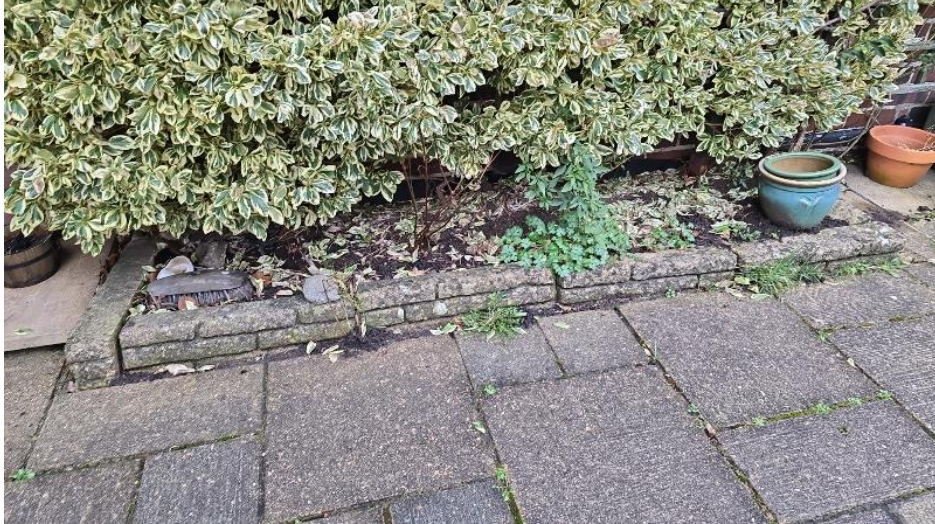
Vegetation to be removed where growing against walls. Raised beds to be removed
