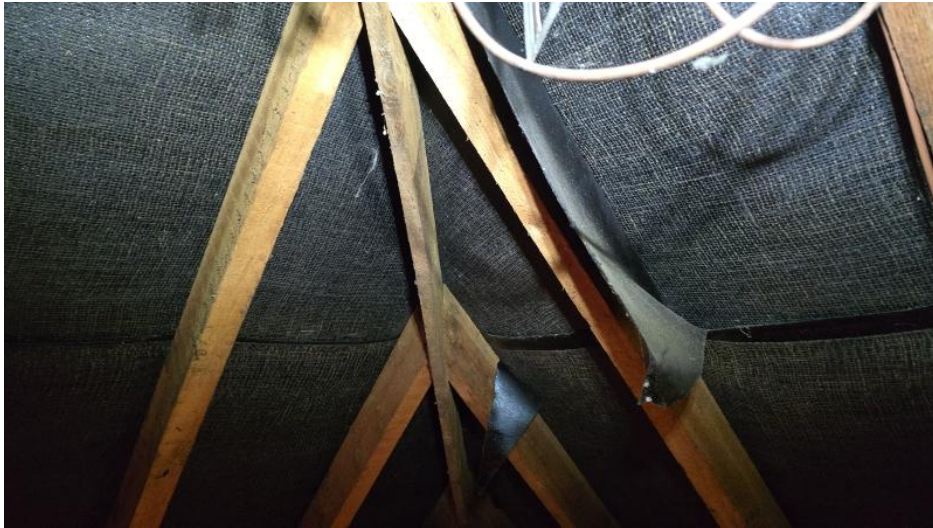
Tear to roofing felt
