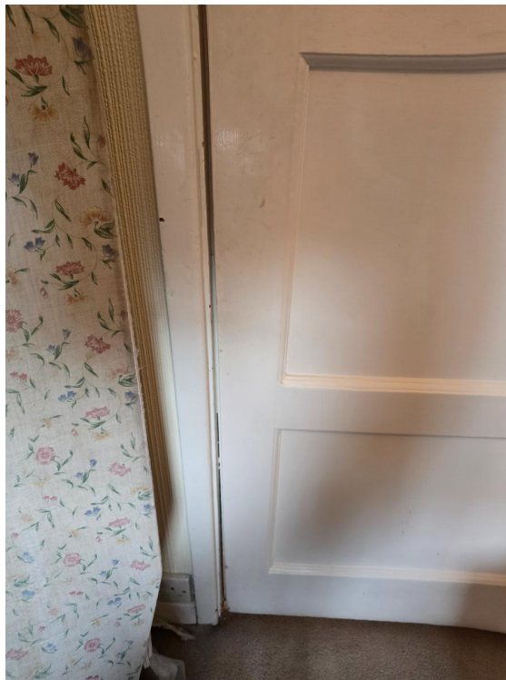
Excessive gaps to bedroom door replace
