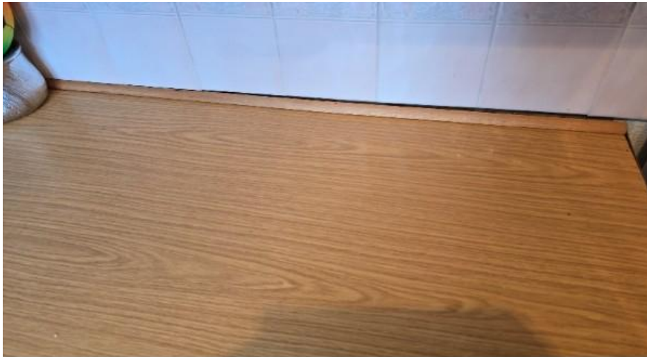
Damaged quadrant beading to utility worktop
