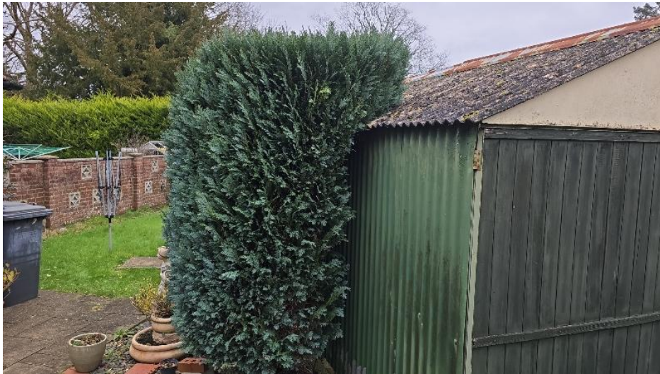
Asbestos roof in poor condition
