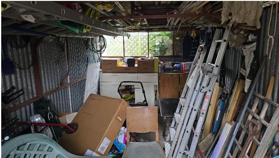
Store items and corrosion to steel frame and fixings
