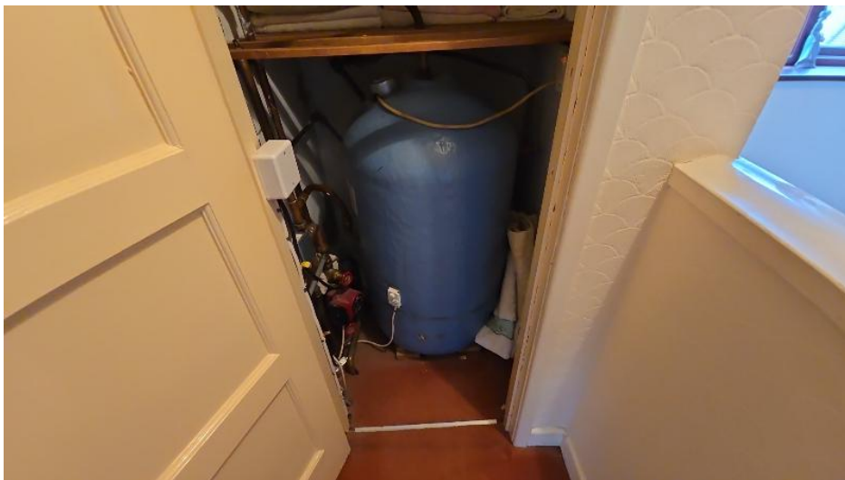
Existing hot water cylinder
