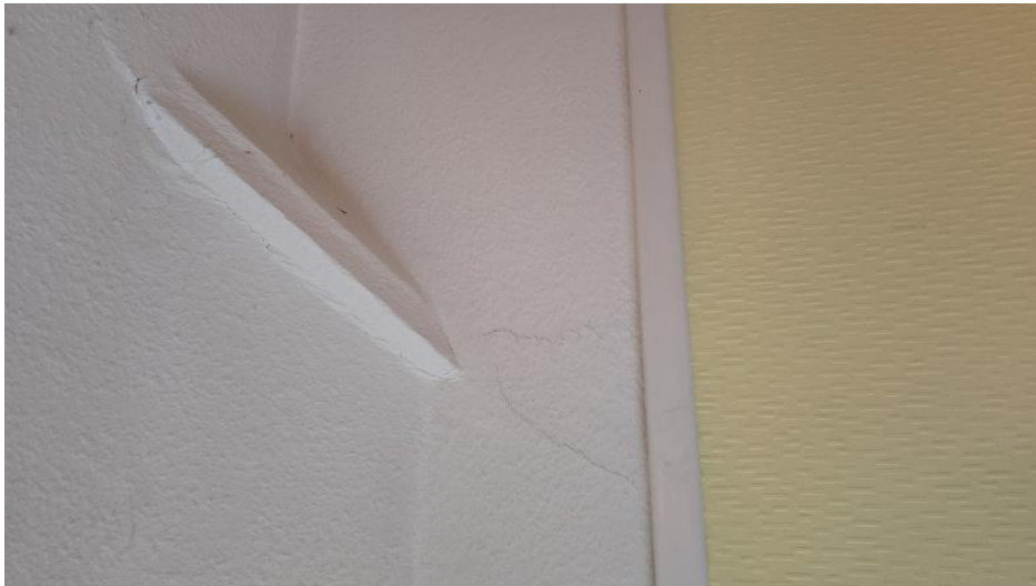
Cracking to wall in Bedroom 1
