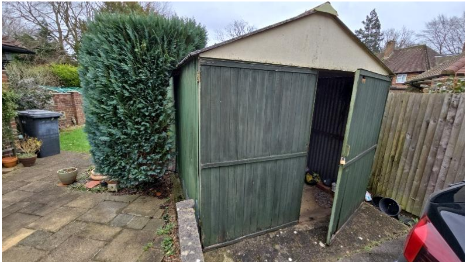
Garage in poor condition
