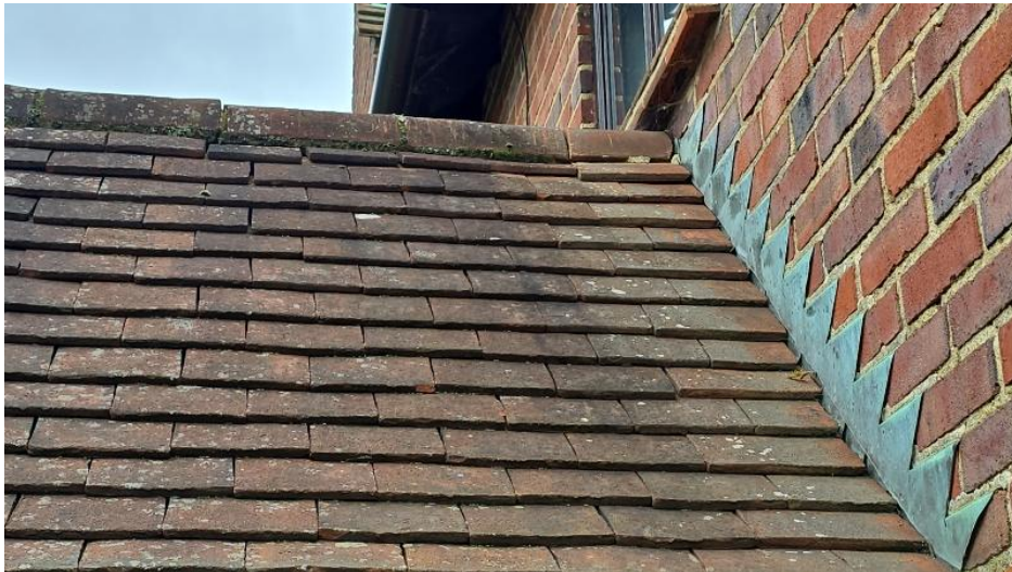
Ridge and roof repairs required
