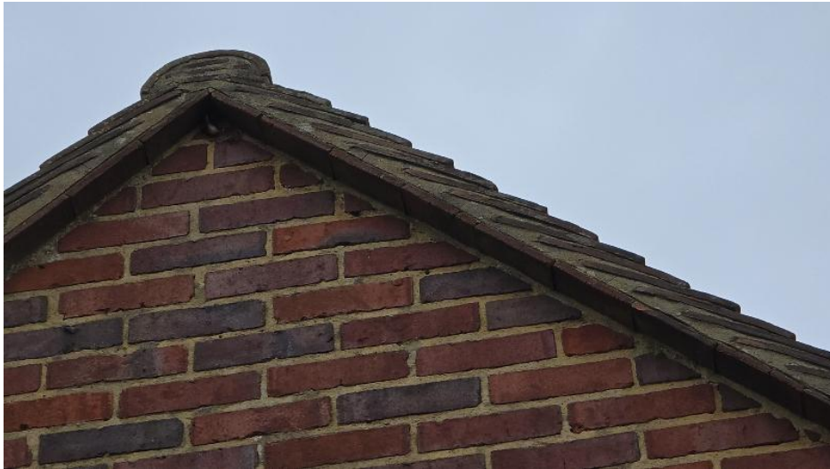
Cracking to mortar on verge
