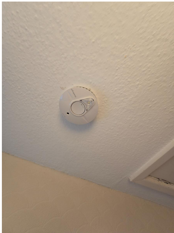
Battery powered smoke alarm 1st floor landing
