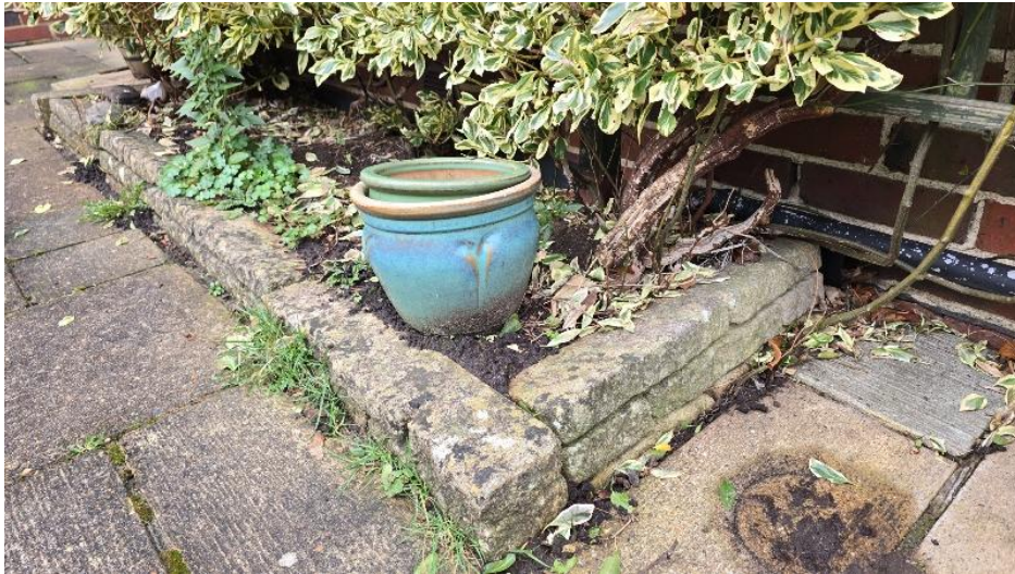
External ground level off rear needs reducing
