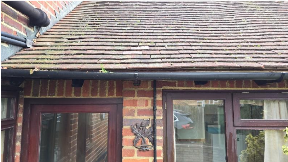
Defective timber to eaves
