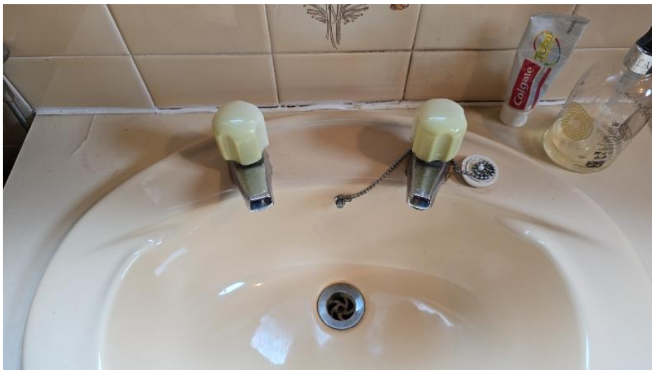
Defective sealant to wash hand basin and damage to countertop
