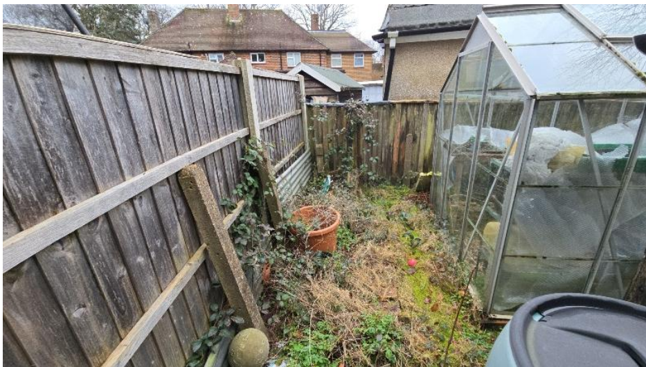
Damaged section of fencing to rear of garden
