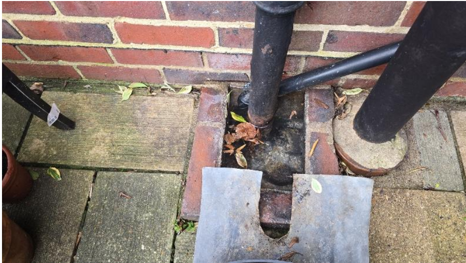
Utility room gully blocked and overflowing
