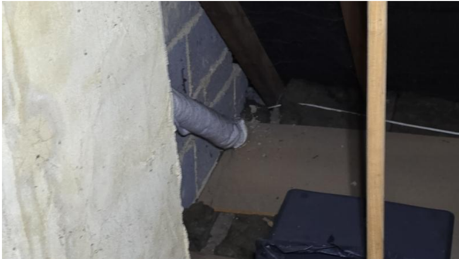
Incomplete party wall
