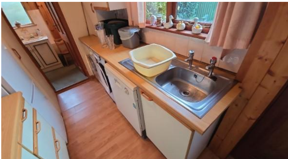
Damaged quadrant beading to utility worktop
