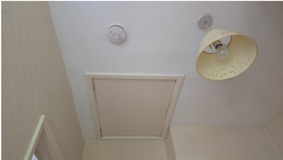
1st floor battery smoke alarm
