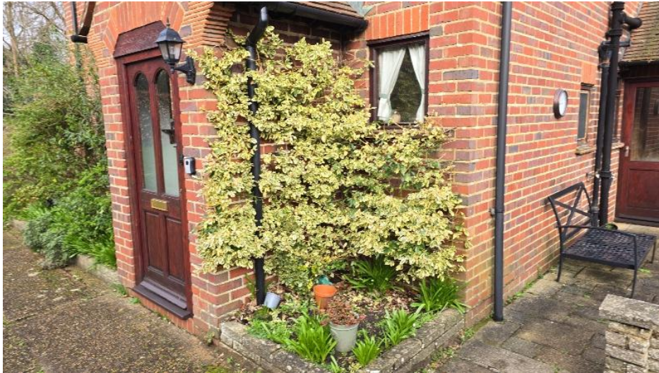
Vegetation restricting our inspection
