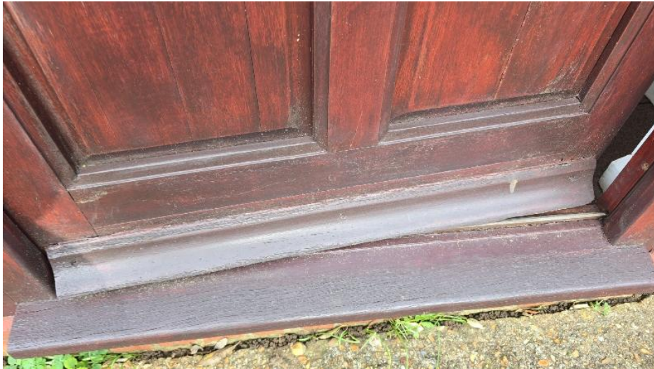
Repairs and redecoration required
