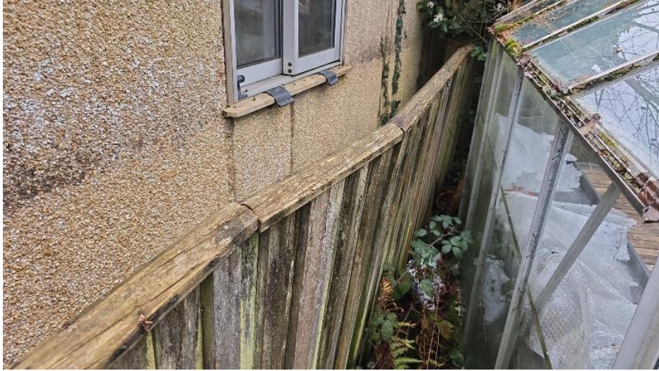
Damaged section of fencing to side of garden
