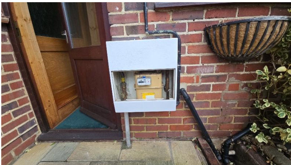
Gas meter with damaged access door
