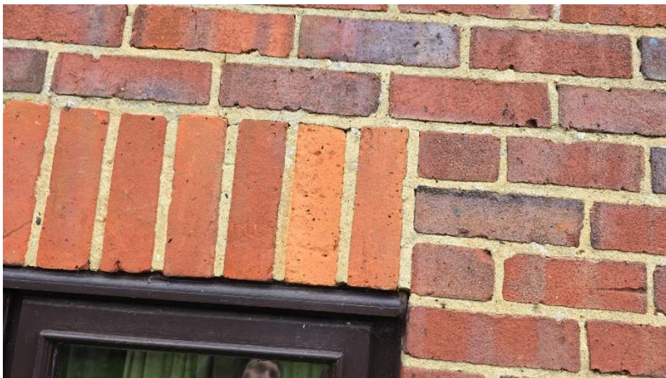
Minor crack above living room window
