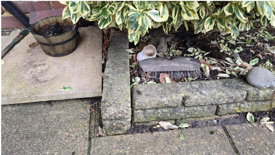
Vegetation to be removed where growing against walls. Raised beds to be removed
