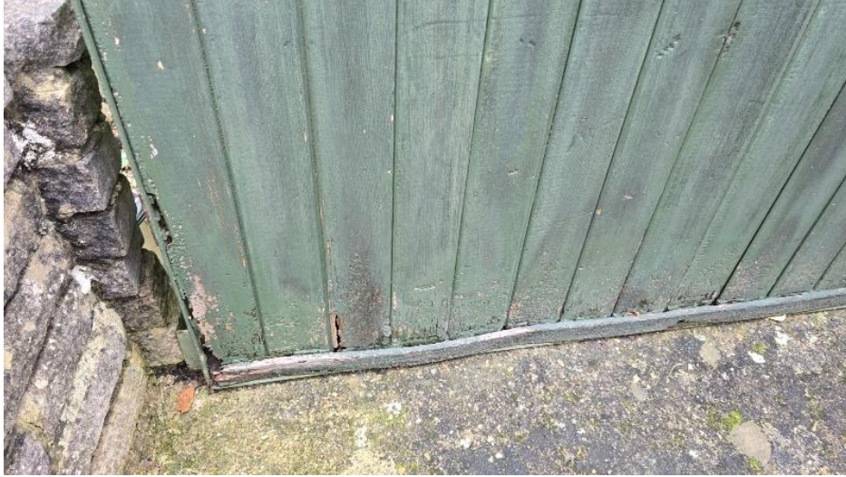
Rotten timber doors
