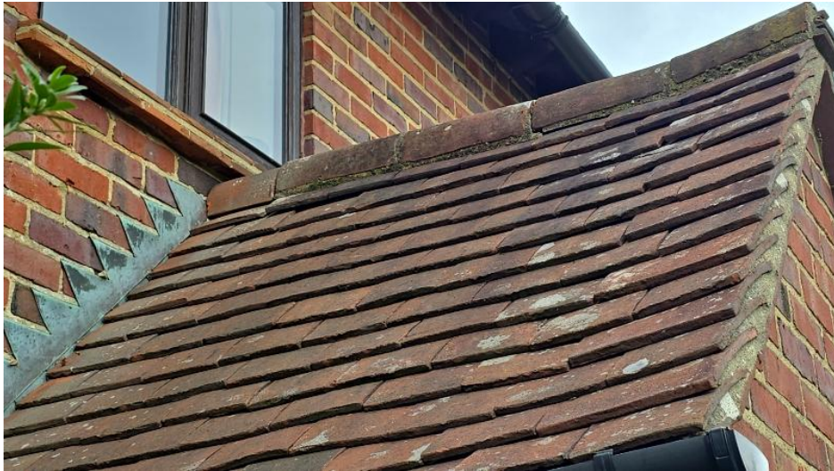
Undulation of porch ridge inspect when replacing tiles
