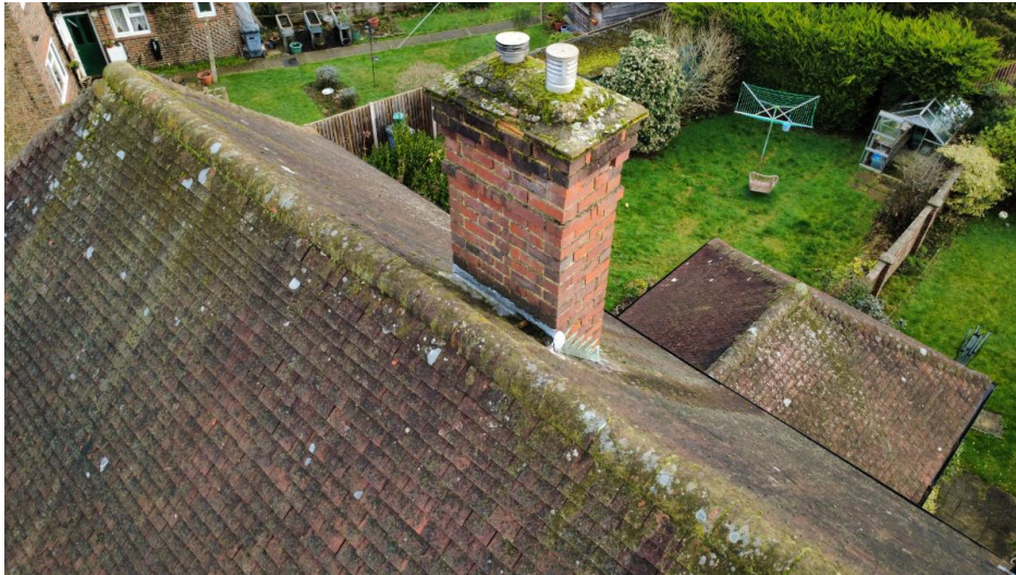
Flaunching replacement required
