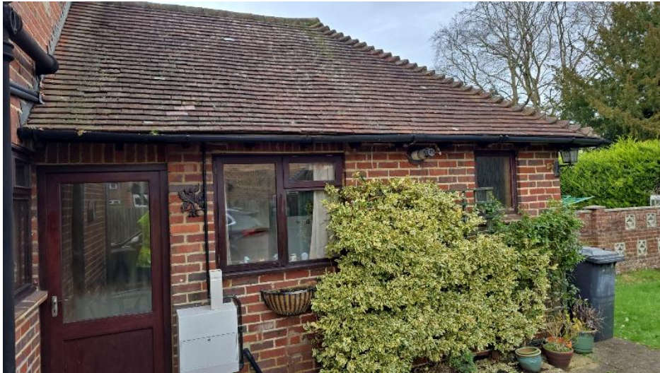
Undulation in gutter due to defective timber to eaves
