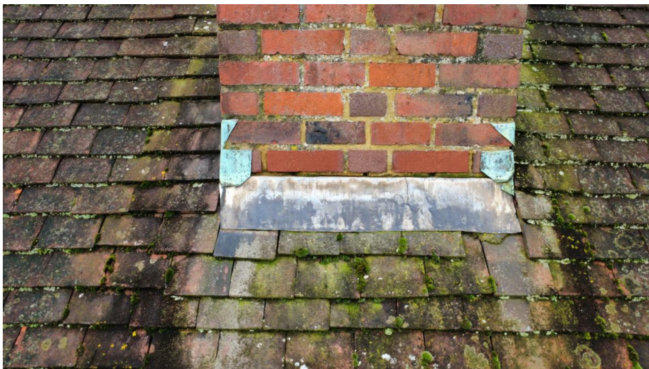
Split lead front apron and missing pointing
