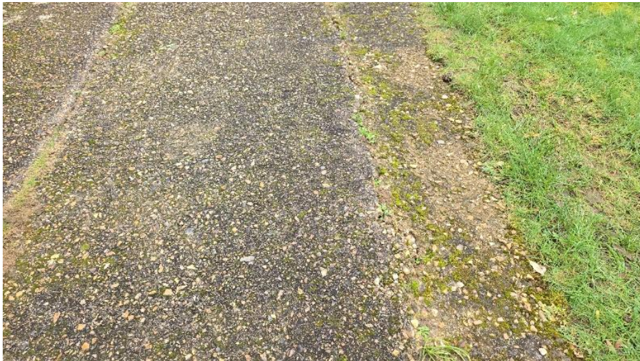
Driveway repairs required
