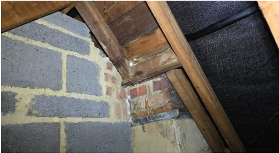
Incomplete fire compartmentation party wall to roof void
