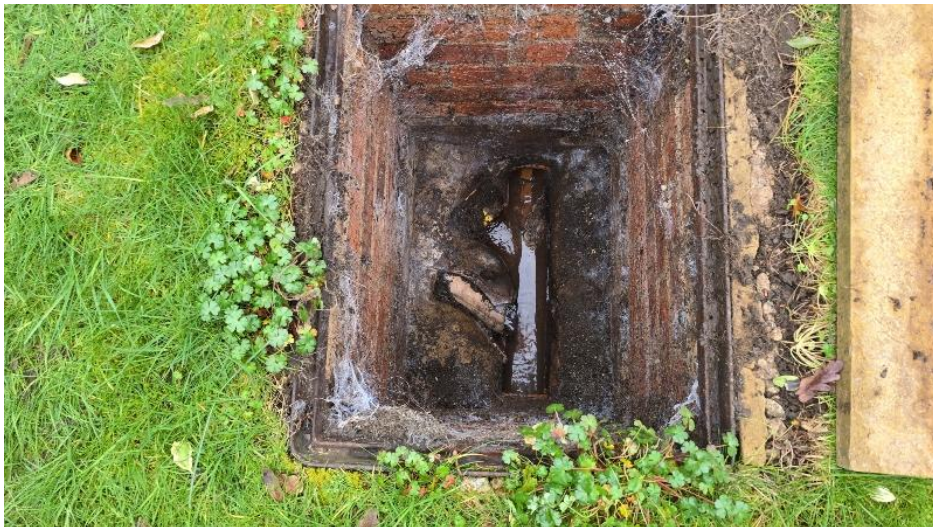
Manhole appears to be clear although detritus and cobwebs restricted the inspection
