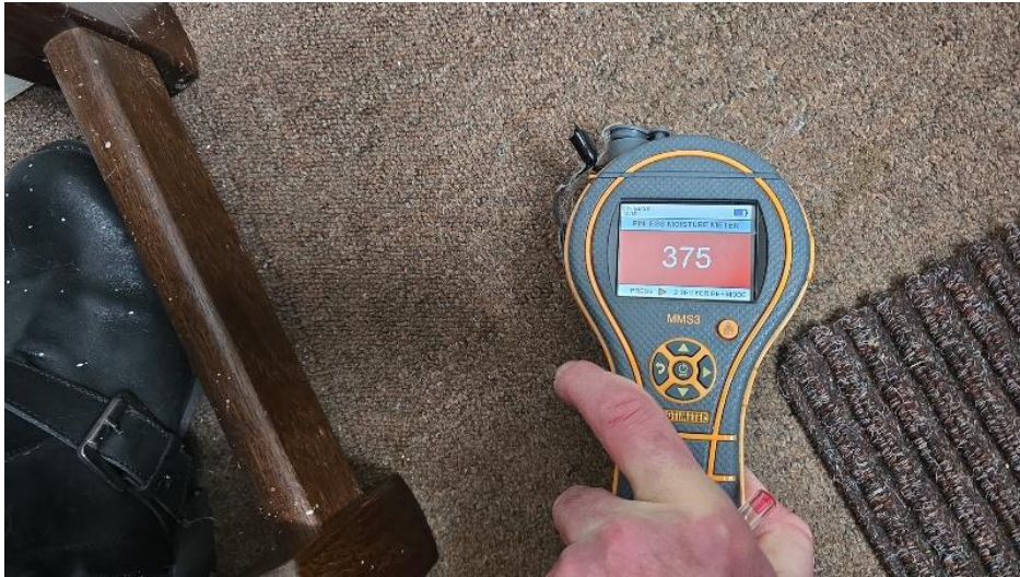
Damp readings to porch floor
