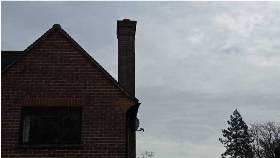
Slight lean towards top of chimney
