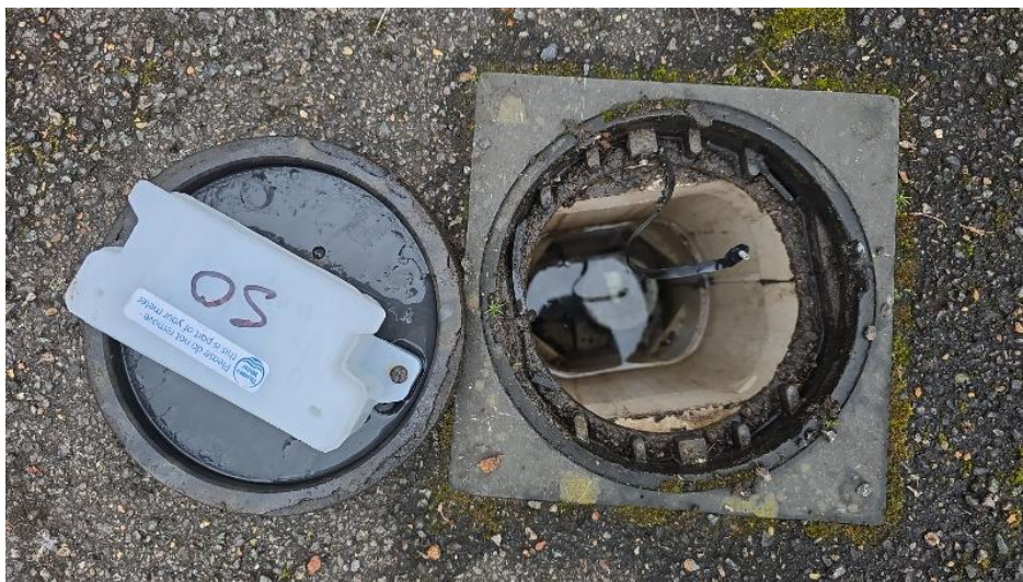
Water meter and external stop valve
