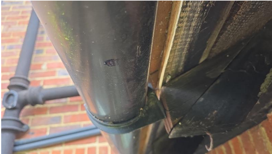
Gutter bracket fixing loose due to defective timber
