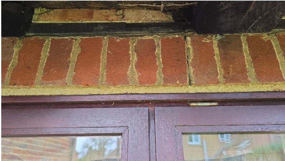
Cracking above utility window lintel
