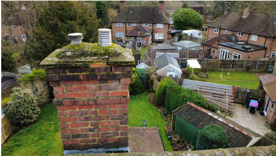
Crack to side of chimney requiring urgent investigation
