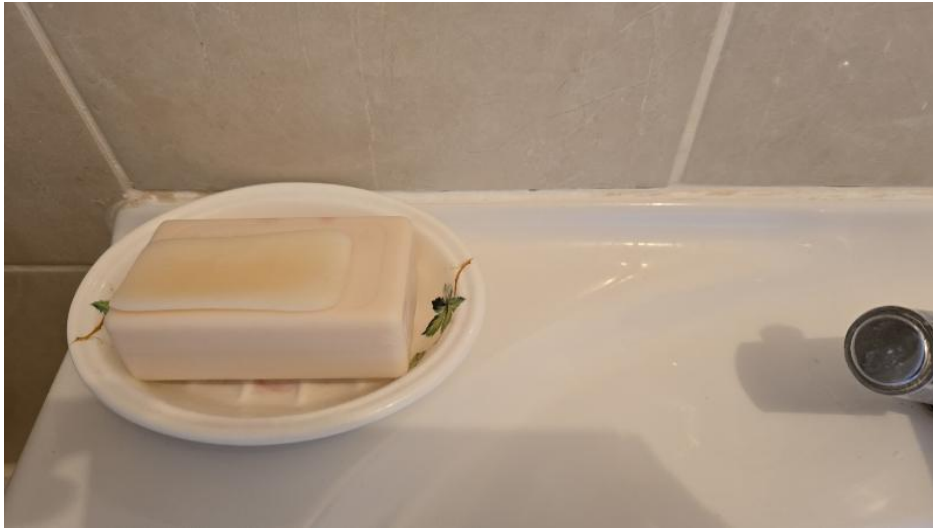
Defective sealant to wash hand basin
