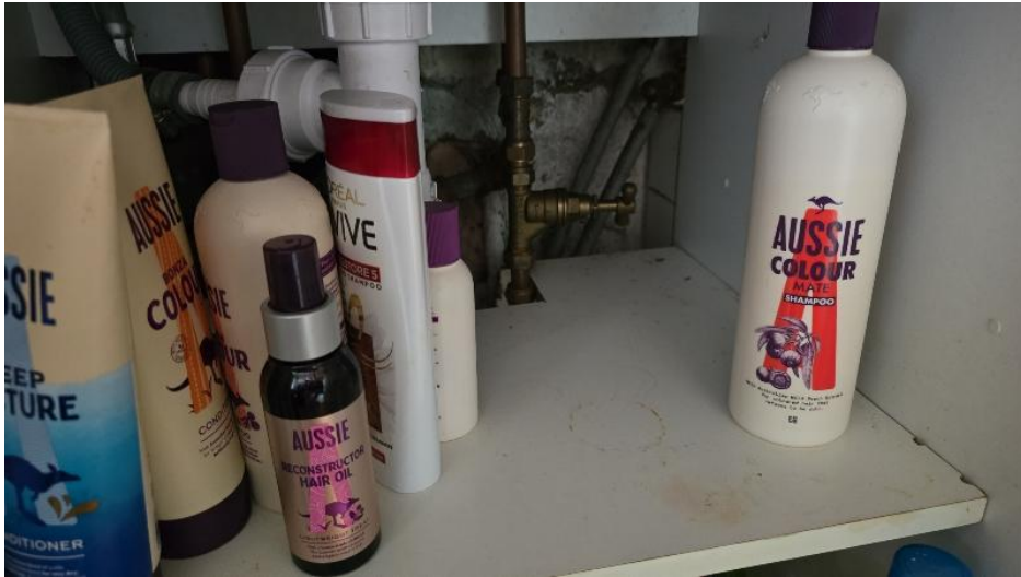
Kitchen sink isolation valve
