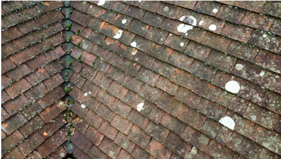
Spalled concrete tiles and debris to gutter
