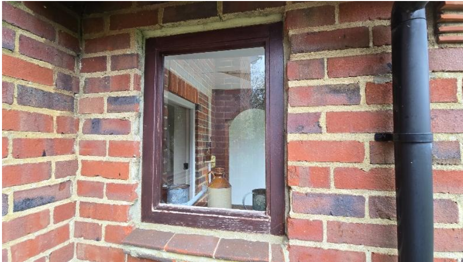
Recent repairs around window
