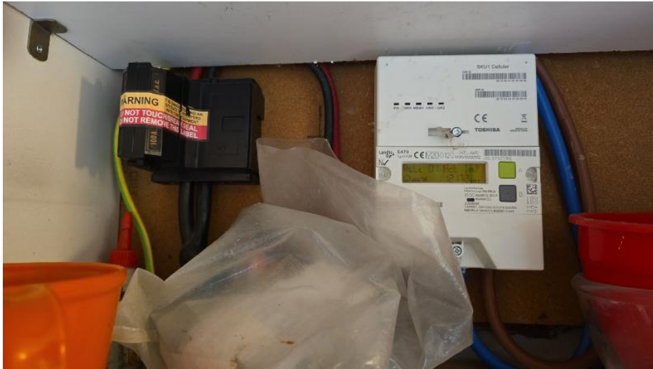
Electrical main fuse and meter utility cupboard
