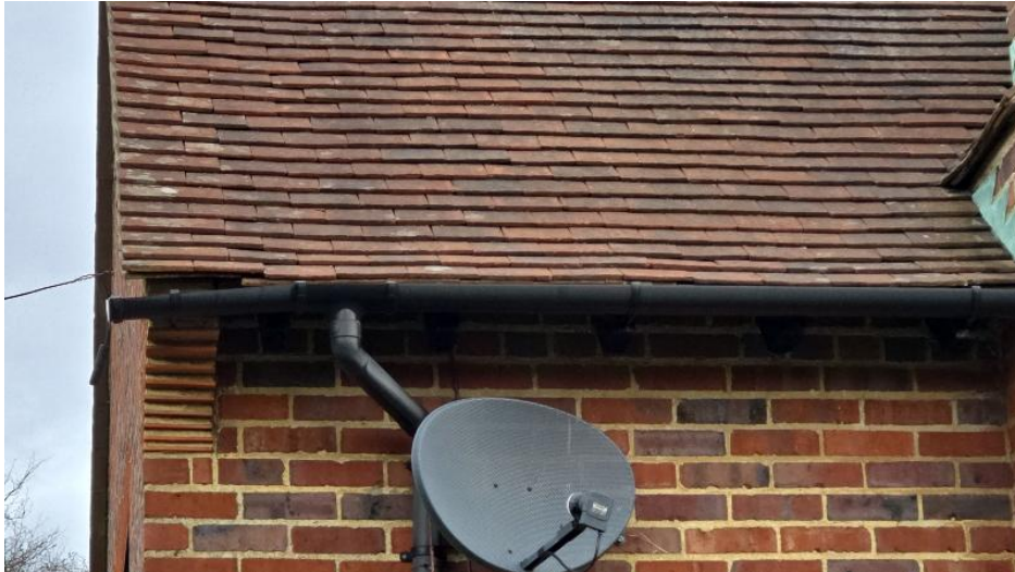
Defective timber at eaves and disconnected gutter bracket
