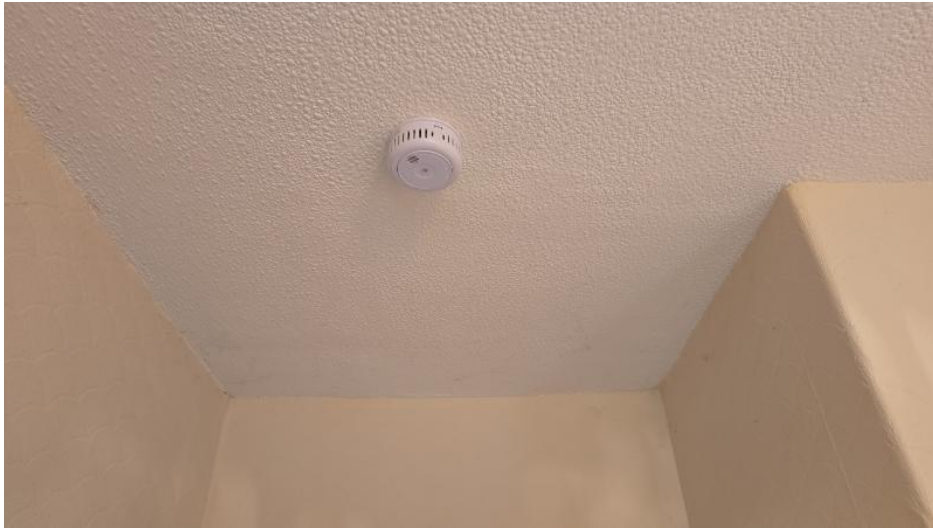
Ground floor battery smoke alarm
