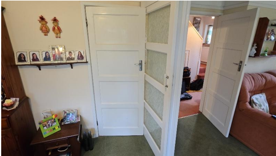
Dining room sliding glazed doors clash with kitchen door. Need to rectify
