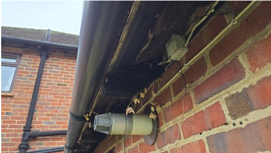
Boiler flue close to underside of roof timbers
