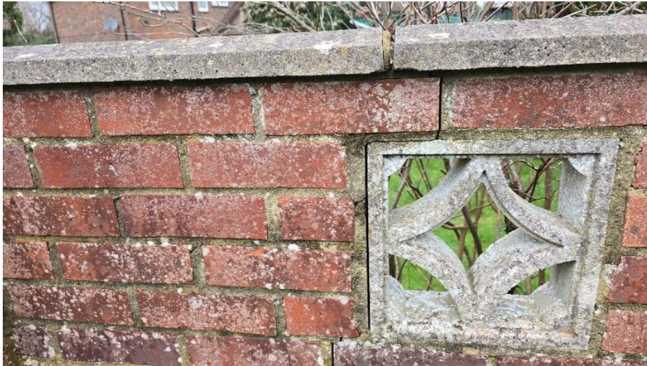
Cracks to boundary wall full height. Further investigations
