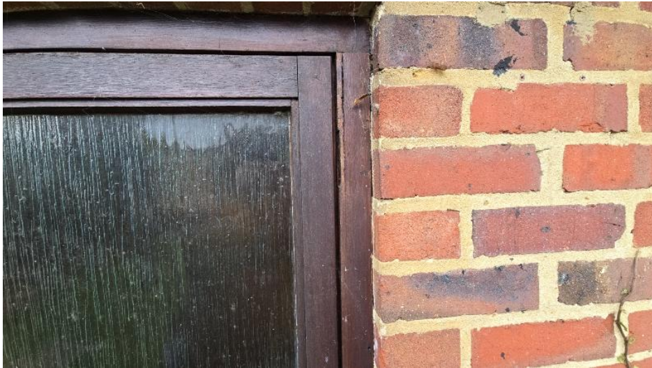
Damaged frame ground floor WC window
