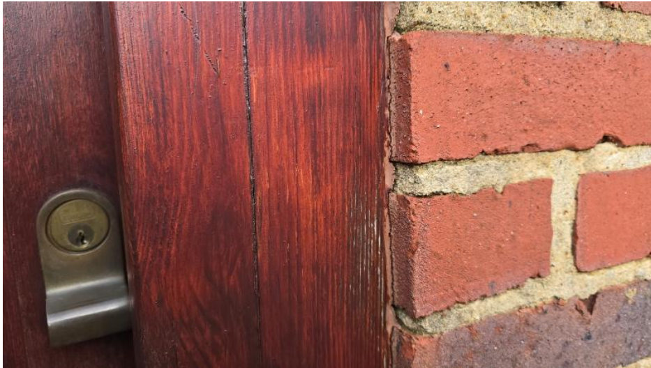
Mastic sealant replacement required
