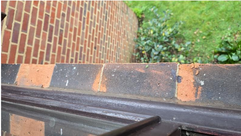
Spalling creased tile to front bedroom window
