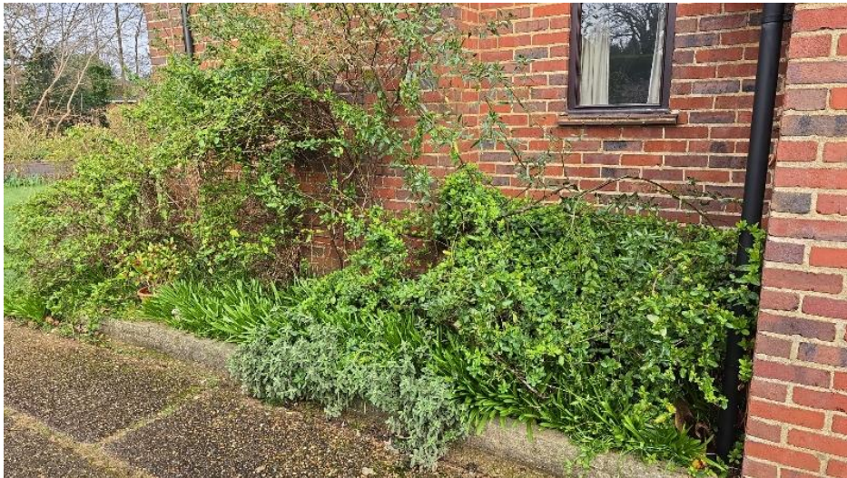
Vegetation restricting our inspection
