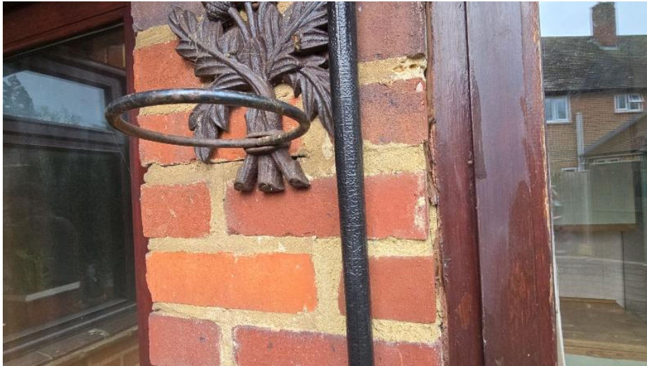
Failed mastic sealant to kitchen
