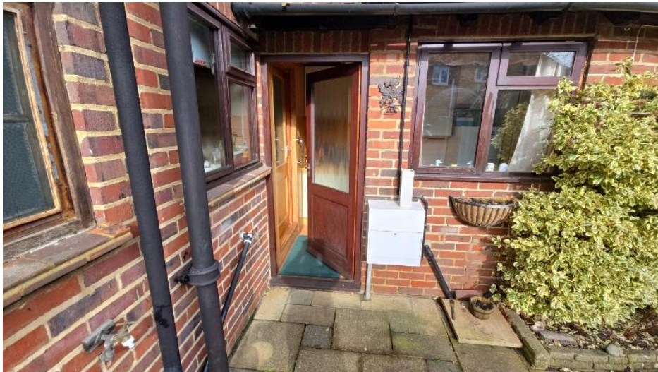
Repairs and redecoration required
