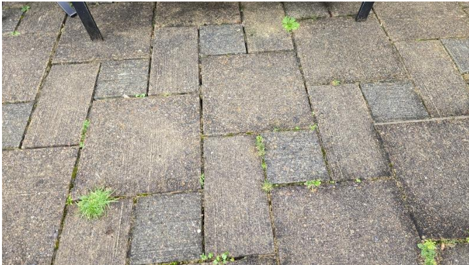
Repairs required to patio
