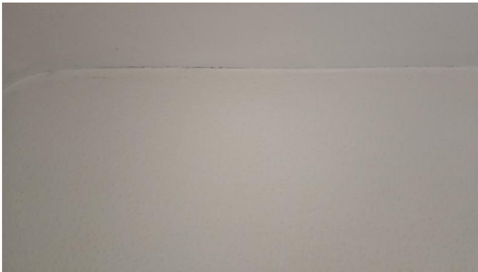
Minor cracking ceiling bedroom 2
