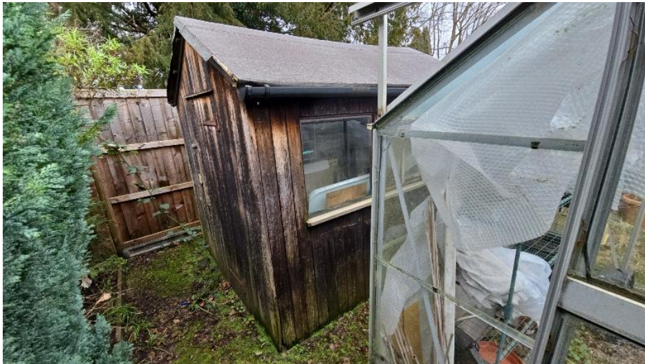
Dilapidated shed no access
