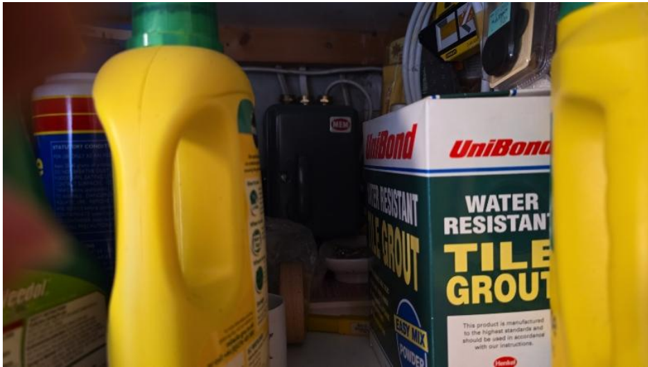
Electrical switch isolator concealed in utility cupboard
