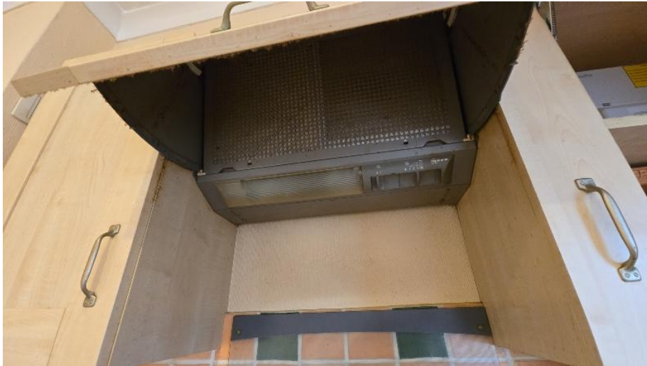
Confirmation as to whether extractor hood is vented due to gas appliance
