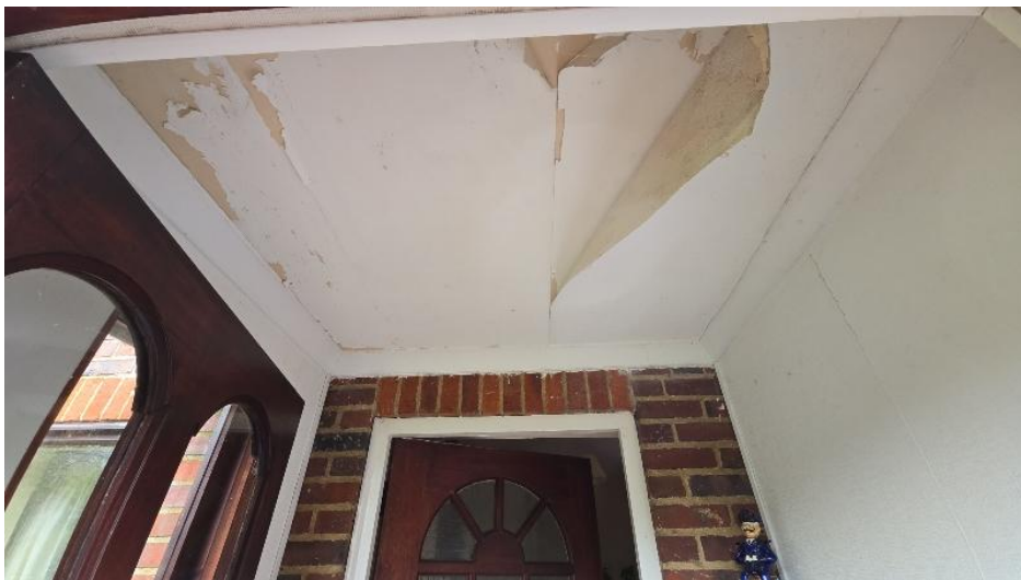
Condensation to ceiling in Porch
