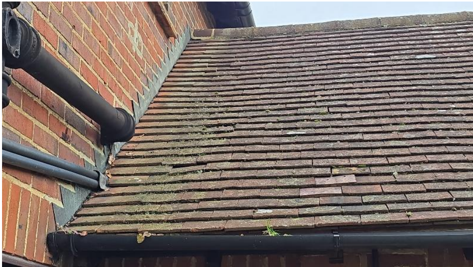
Slipped and missing tiles to utility room roof
