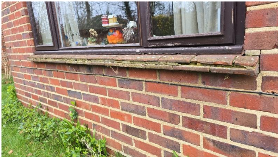
Repairs or replacement of creased tiled Living room window cill
