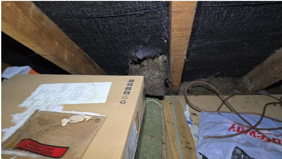
Tear to roofing felt
