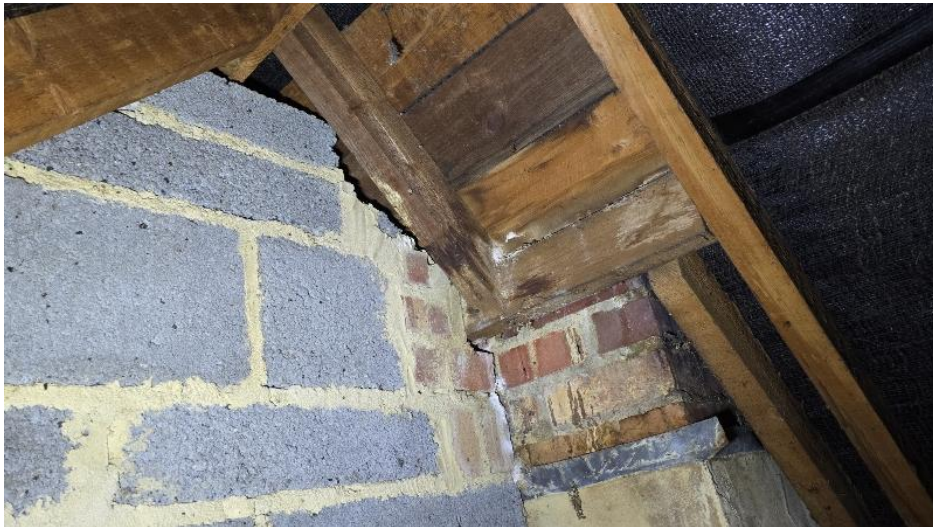
Incomplete party wall and rot to chimney timbers
