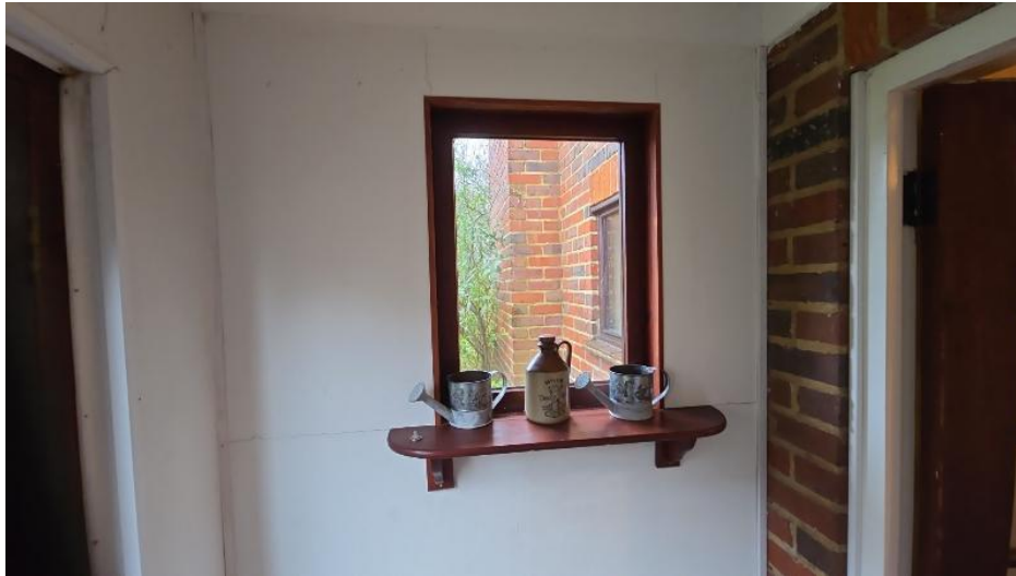
Cracking dry lined walls
