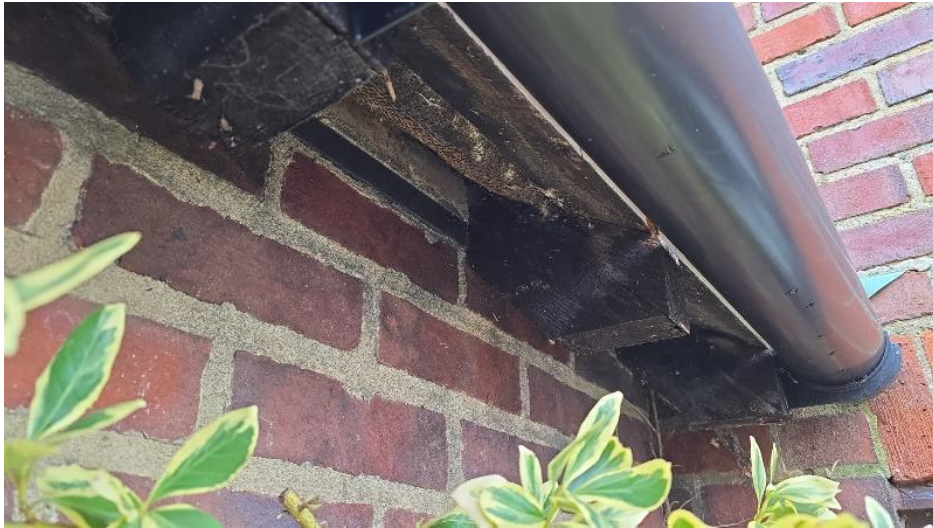
Defective timber to underside of eaves
