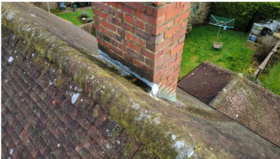
Debris and poor detailing to back gutter
