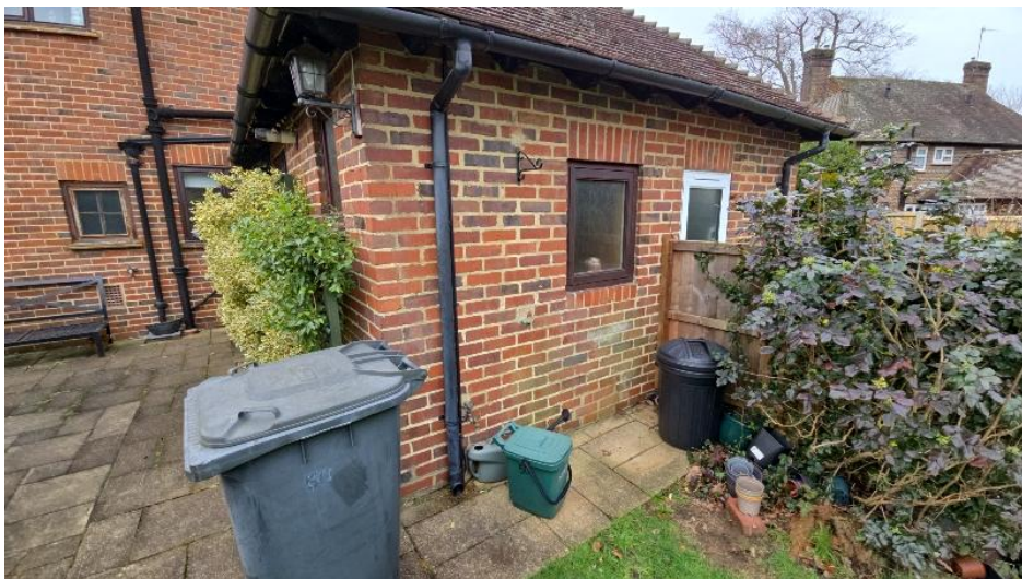
Alterations to existing gutters. Downpipe discharges directly to ground
