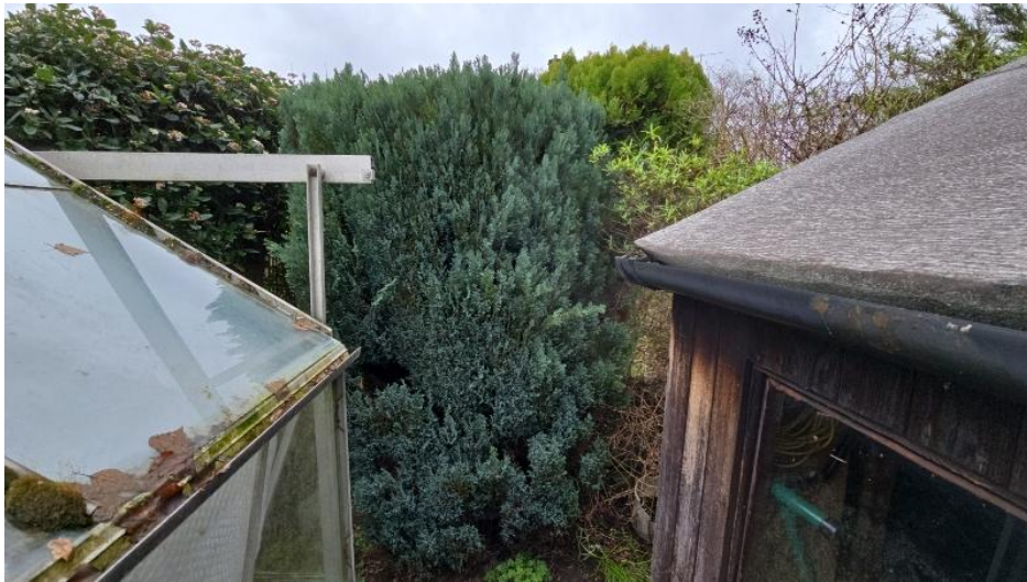
Vegetation growth limiting inspection
