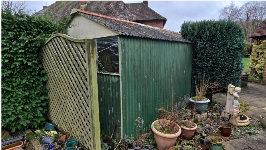
Asbestos roof in poor condition
