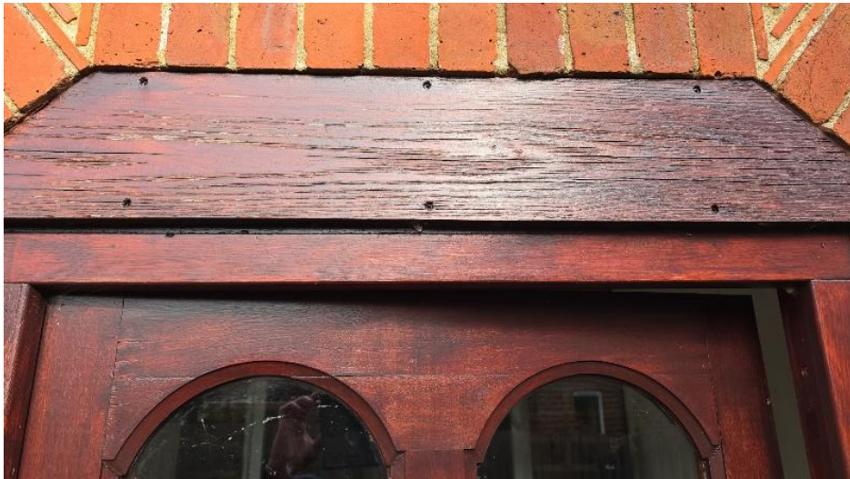
Repairs and redecoration required
