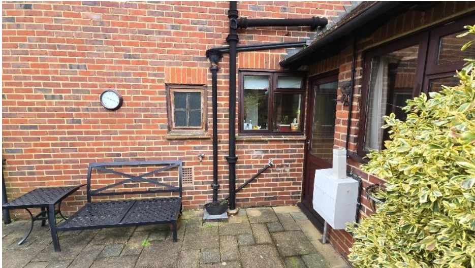
Cast iron downpipe and hopper repairs required
