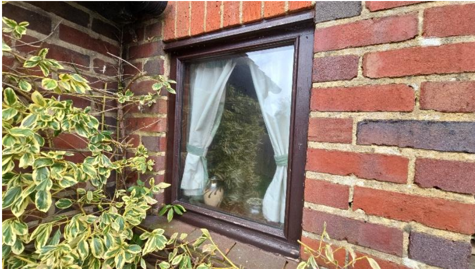
Failed double glazed seal units stairs window
