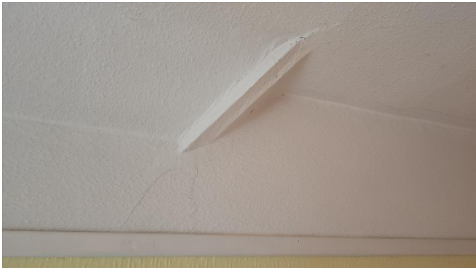
Cracking to ceiling around roof timbers in Bedroom 1
