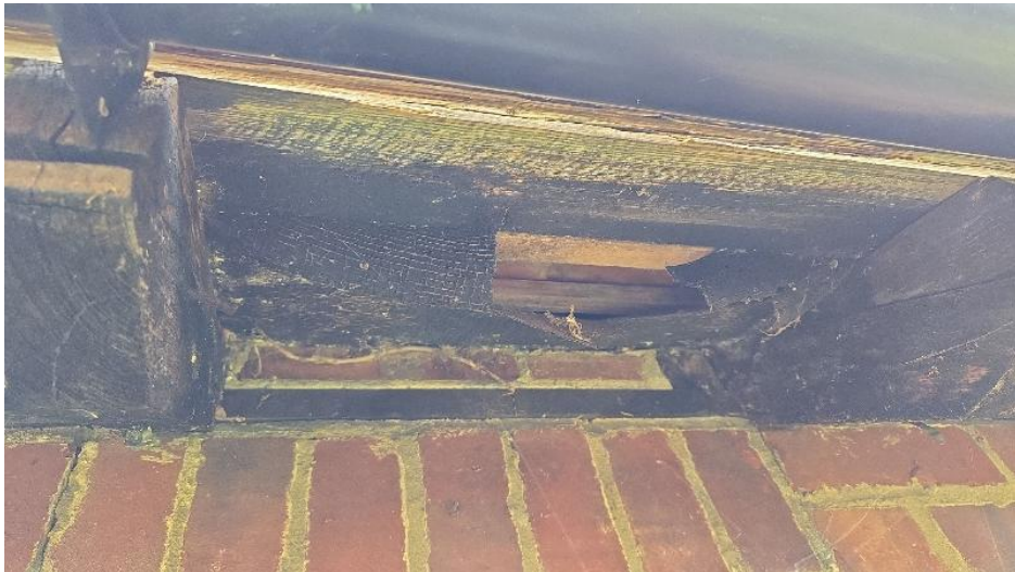
Defective timber to eaves
