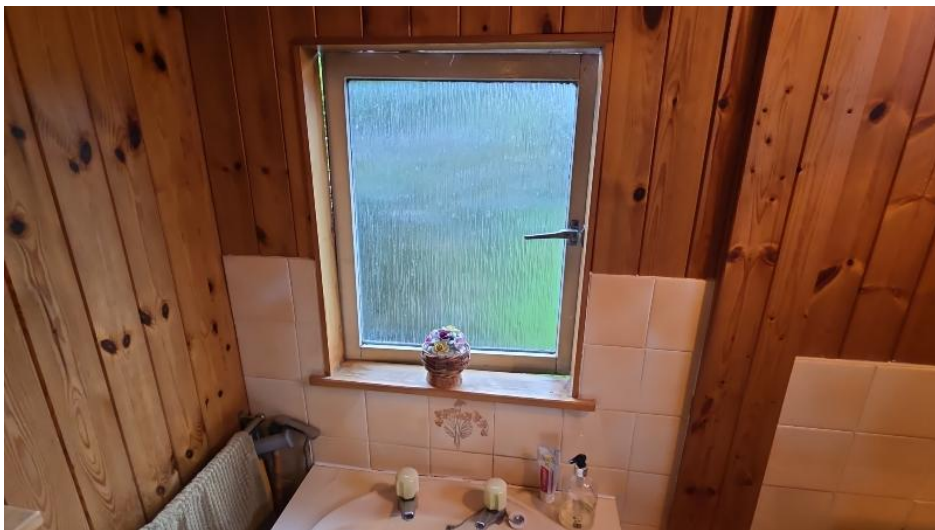
WC window frame broken and doesn't fully open
