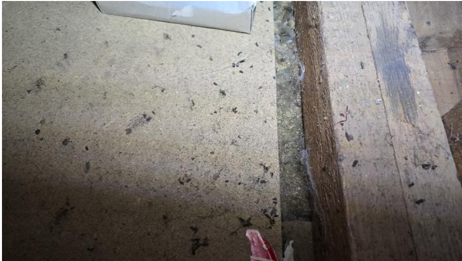
Vermin faeces and evidence of wood boring insects
