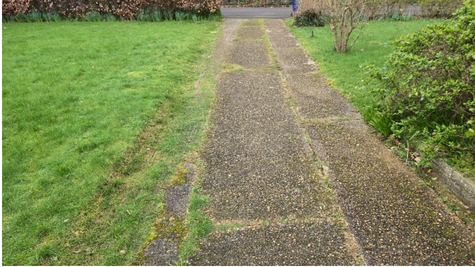
Driveway repairs required
