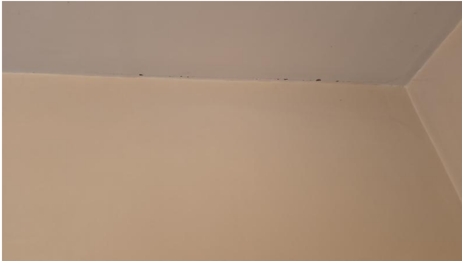
Cracking to ceiling in bathroom
