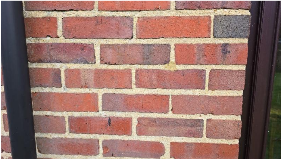
Typical mortar repair following retrofit cavity wall insulation
