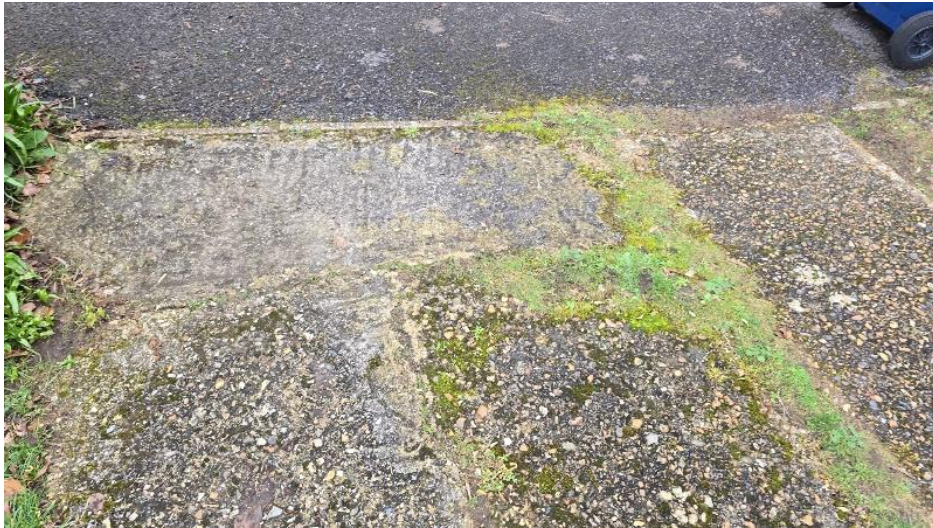
Driveway repairs required
