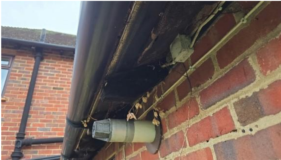
Non condensing boiler flue close to eaves and guttering
