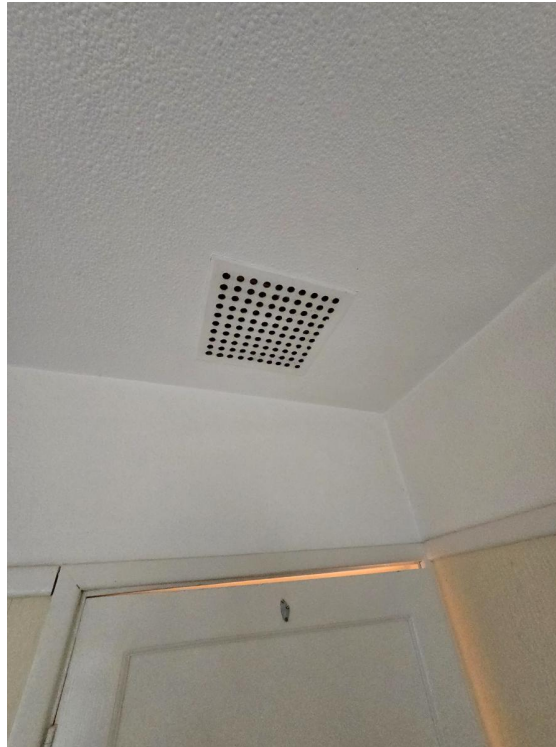
Old presumed warm air vent ducts located throughout the property.
