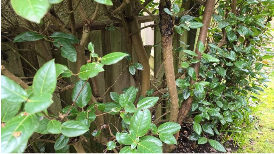
Damaged fence behind vegetation
