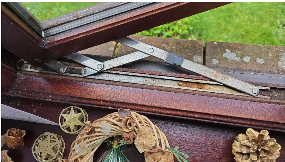
Corrosion to ferrous fixings
