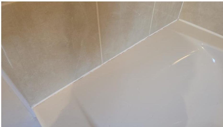
Defective sealant to bath
