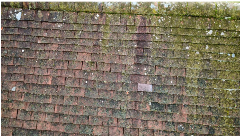
Moss growth, slipped and missing tiles
