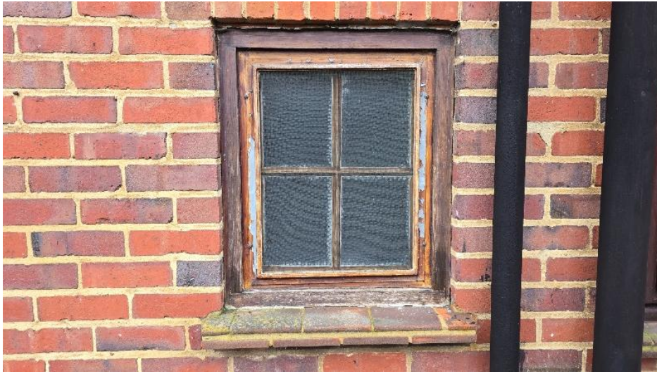
Metal single glazed window to larder
