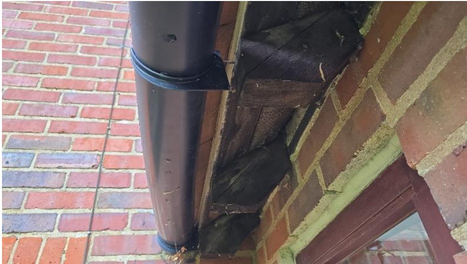
Torn underlay to eaves, defective timber
