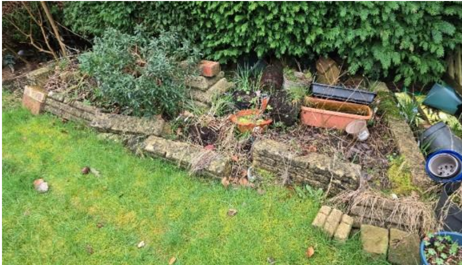
Dilapidated section of low level wall/raised bed to be rebuilt
