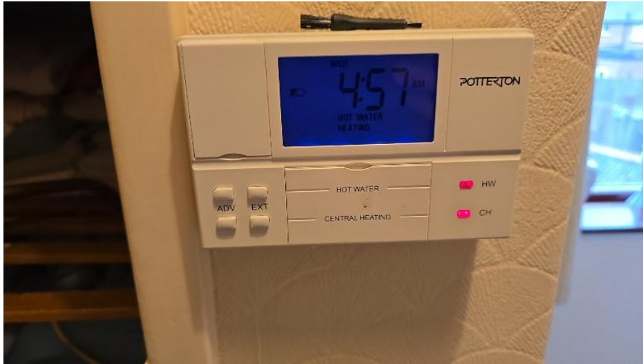
Heating and hot water timer
