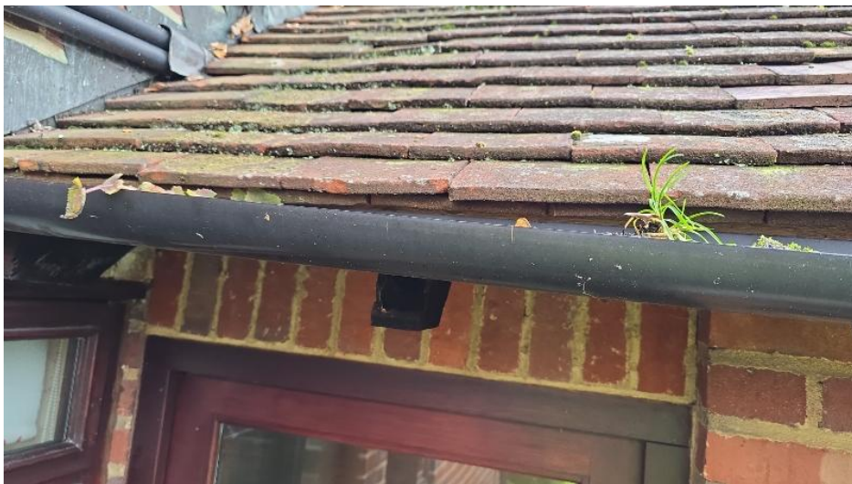
Displaced gutter as a result of defects to roof timber
