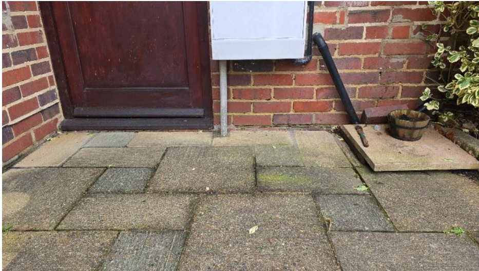
External ground level off rear needs reducing
