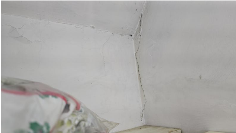
Cracking to external airing cupboard wall
