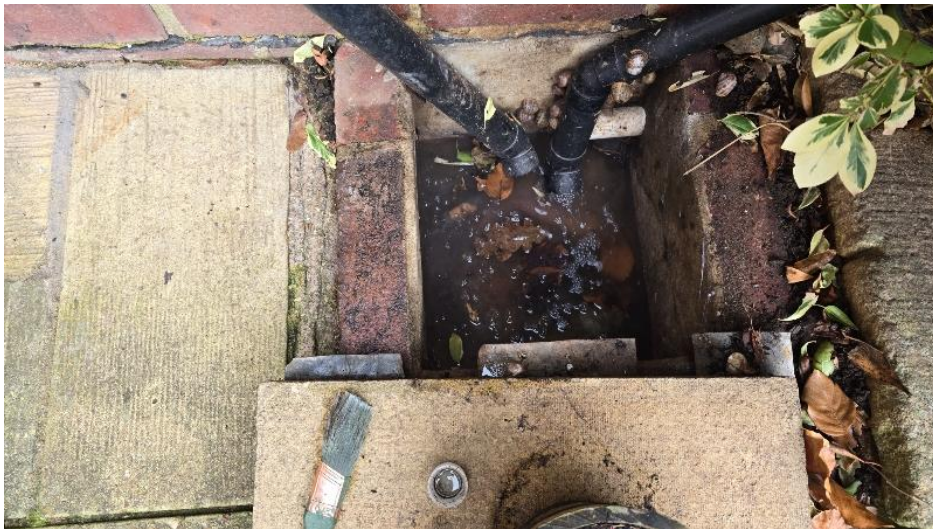
Kitchen gully blocked and overflowing
