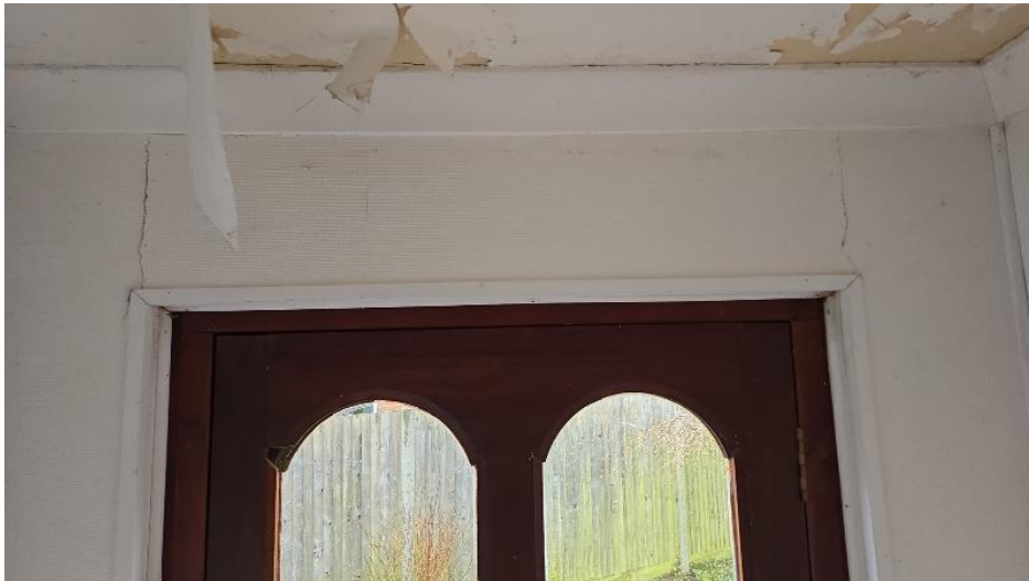
Cracking dry lined walls above door
